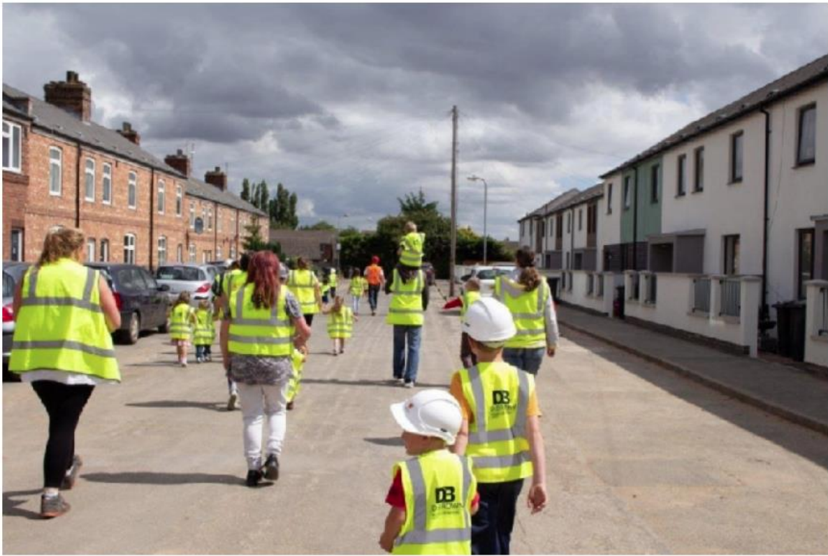
Old and new homes on Newfield Road during the initial phases of work. EMN-190618-174231001
